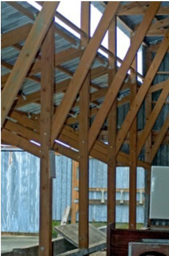
The project included new posts and braces to support the main trusses and east roof overhang. Photo by Georgette Ferdun
