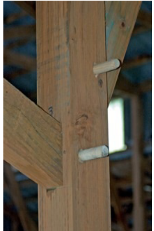
Traditional timber frame construction was used for the barn repair utilizing trenails and mortise and tenon joinery. Photo by Gareth Ferdun
